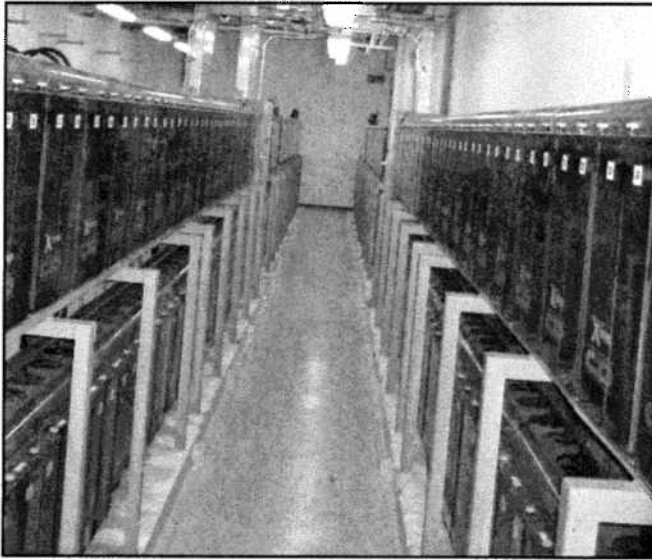
Fig. 7 Picture showing the two tier single row flooded battery strings with spill containment.
