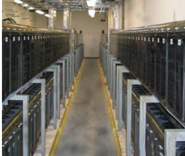
Before: Lead Acid (Flooded)
